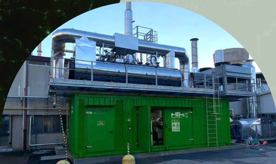
Natural gas plant in Grandate (CO) 500 kWe electrical power 565 kWt thermal power
